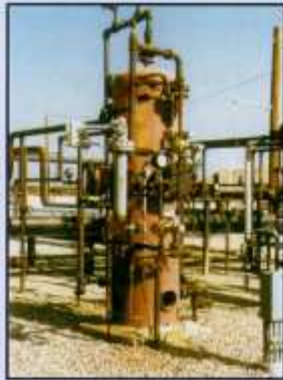
BEFORE: A process vessel with three float switches, two short sight glasses, a pneumatic level controller and 15 valves and associated plumbing.
