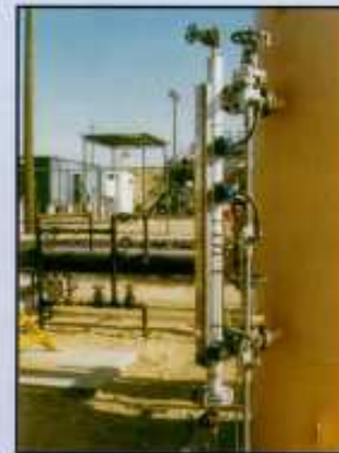
AFTER: The same vessel shown at left after installation of a magnetic gage and the same controls (plus more) at about half the cost to the customer.
